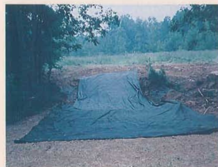
A geotextile fabric will lengthen the life of the approaches and reduce the amount of rock needed. Note the baskets placed on either side of the fabric.
